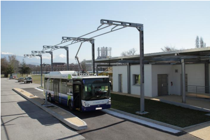
Figure 8: CEA 350kW charge station
