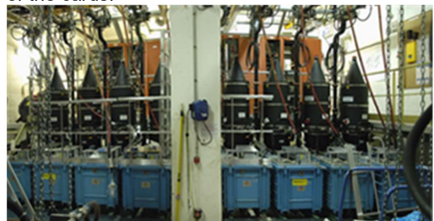
Fig. 8: Implementation of the protection opening switches (in the blue enclosures)
