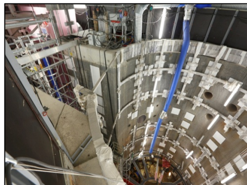
April 2014: Reactor pool internal structures © CEA
