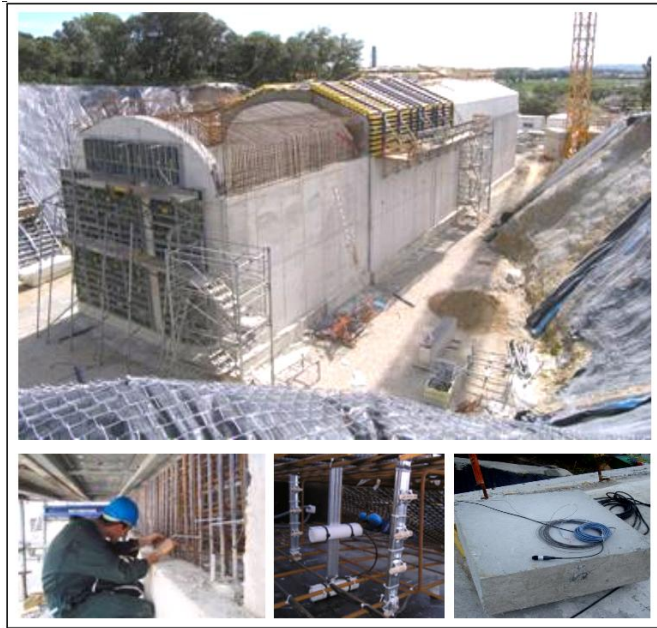
Figure 9 : Overall view during construction of the vault of GALATEE. View of the instrumentation embedded and of the comparison wall built during construction
