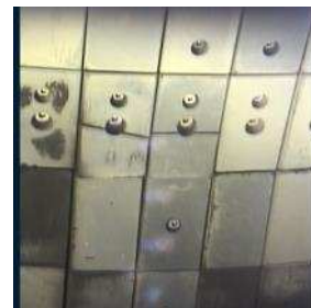
Fig. 7 - Broken tile observed in EAST vacuum vessel [5]
